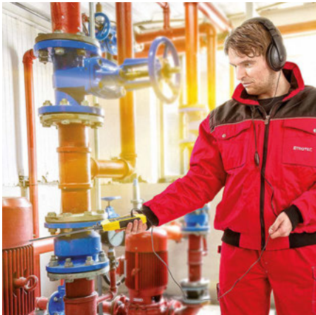
Signs of wear at pumps and other processing machines can be detected at an early stage using the structure-borne sound probe.
